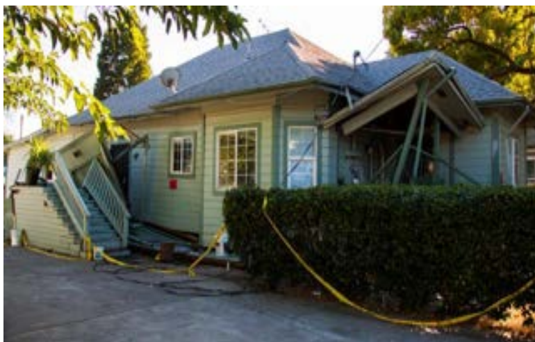
Figure 25 Structural Earthquake Damage
