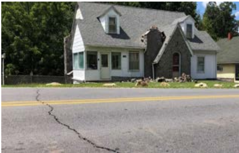
Figure 24 Minor Earthquake Damage
