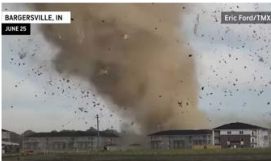
Figure 44 Debris Flying as Tornado Destroys Apartments under Construction
