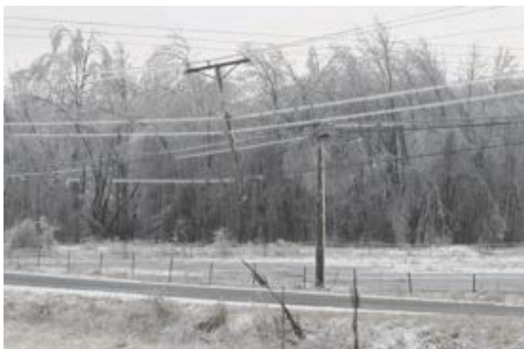
Figure 46 Ice Covered Power Lines
