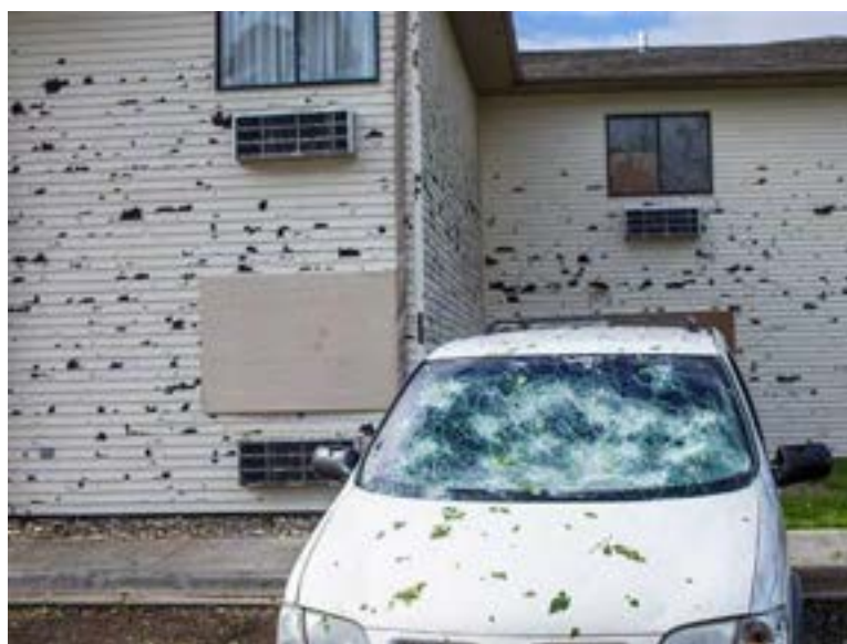
Figure 39 Damage to Vehicle and Structure Caused by Hail
